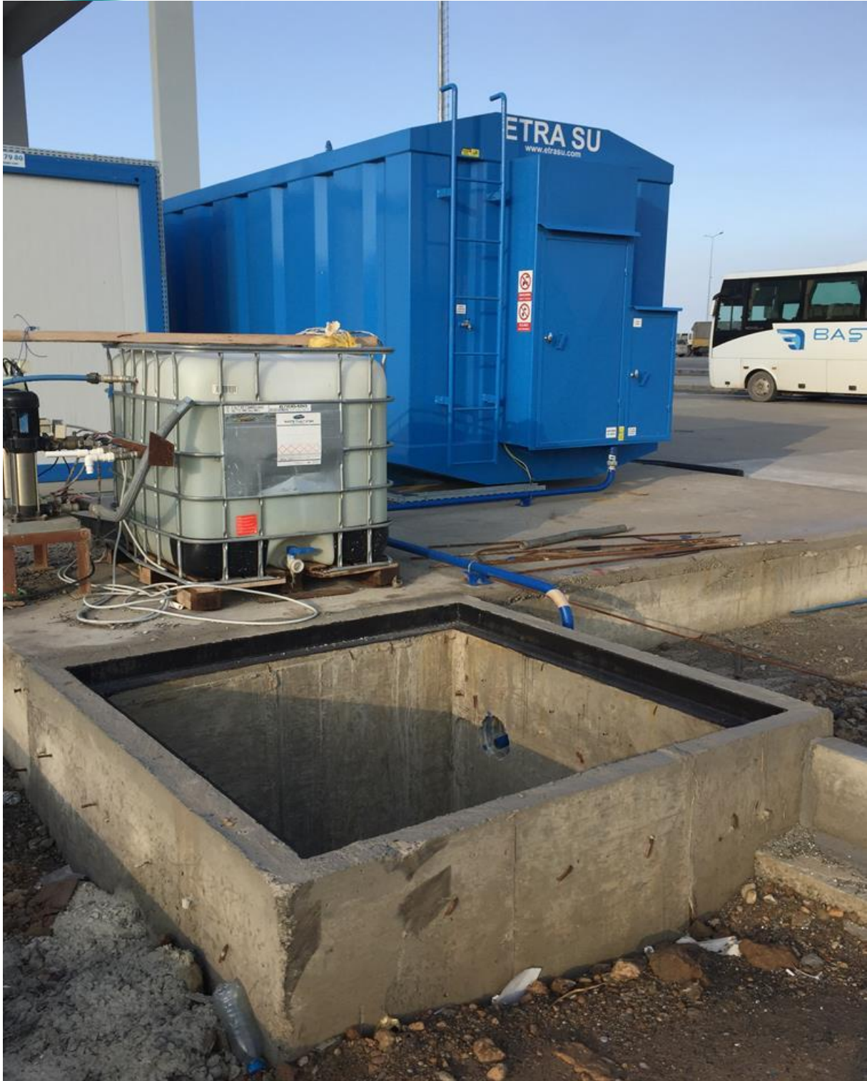
Discharge Manhole and Discharge Water Sampling Point
